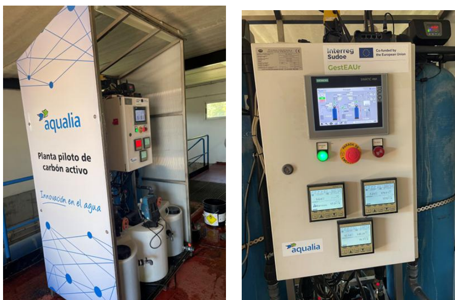
Figure 3. Activated carbon pilot plant in Nogales DWTP (Badajoz, Spain)
