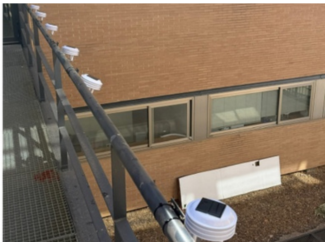
MOX sensor nodes installed at the School of Industrial Engineering for firmware testing.
